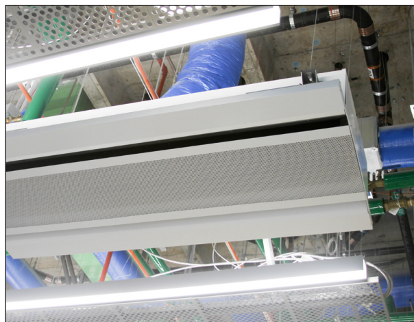
CBLE installed in an open ceiling of a college classroom
